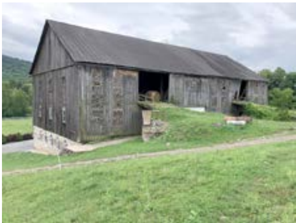
Teachers and soulmates who loved the land, the late Hugh and Barbara Hodge (top) donated an ag conservation easement in 2003 on their 150 acres and historic barn. The double-bank barn as it looked in September 2021 (above) and being repaired in May 2023 (left).
